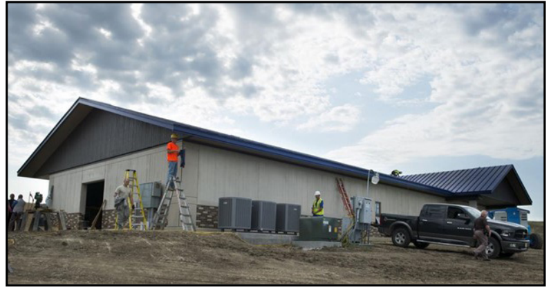
The Lincoln Police Department's law enforcement training campus includes a multi-use building with classrooms.
